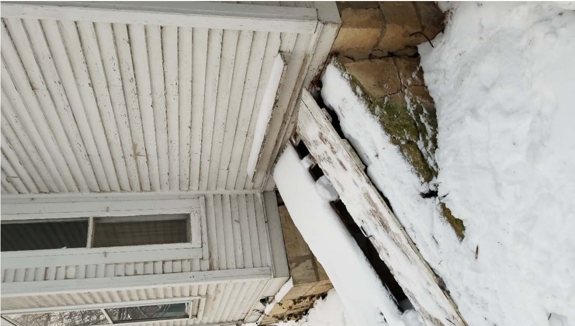
Image 22 – Stone foundation at exterior basement access pulling away and failing.
