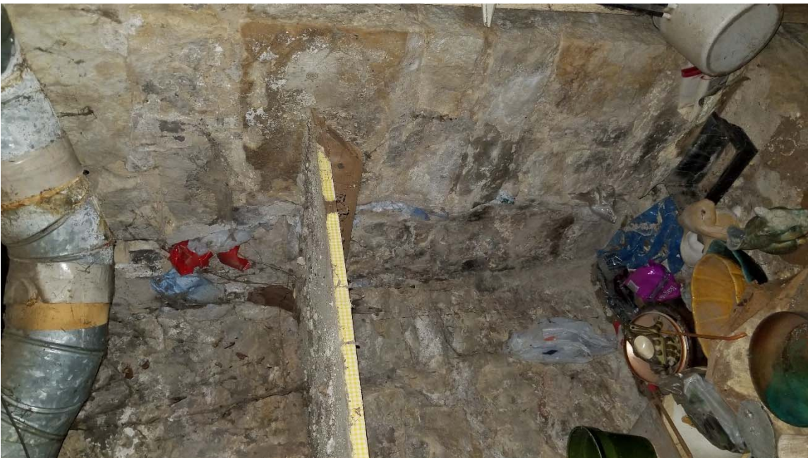
Image 14 – Ductwork is corroding and stone foundation has signs of patching large cracks with plastic bags shoved in cracks and towards bottom one of the cracks appears to be filled with silicone caulk.
