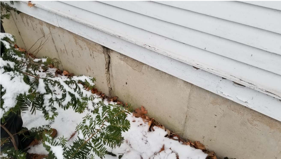
Image 10 – Concrete foundation with significant crack with separation in foundation.
