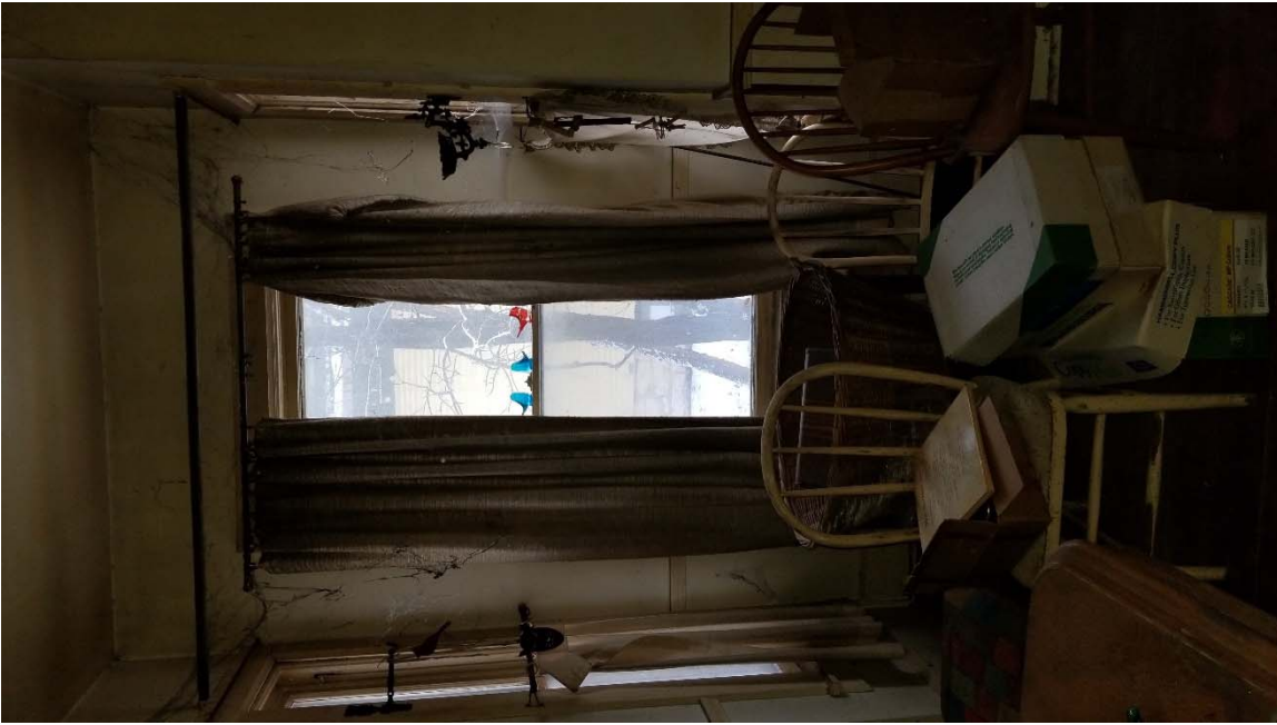
Image 11 – Bay bump out at dining room from inside with floor, walls and ceiling dropping at outside wall.
