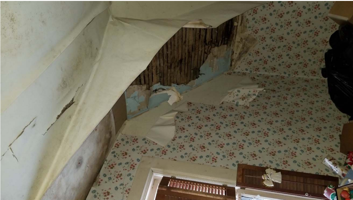
Image 6 – 2 nd floor southeast bedroom with ceiling falling in and showing signs of mold due to water damage
