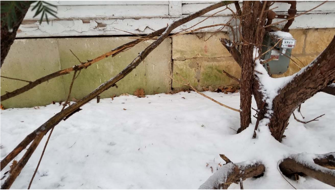
Image 9 – Concrete foundation dropped or settling at stone foundation. Stone foundation has signs of cracking also.
