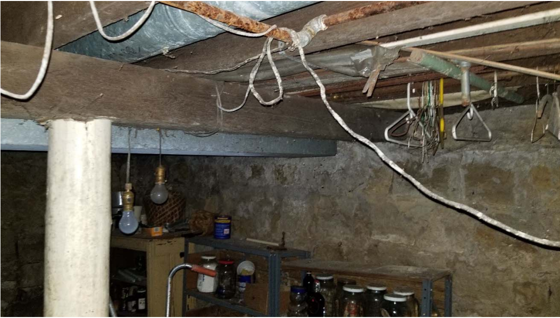
Image 15 – Undersized basement wood beam with lights hanging from ceiling with rope cord
