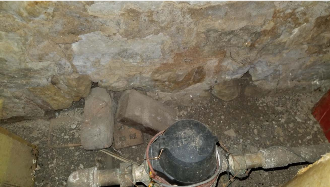
Image 13 – water meeting with copper connections to lead water piping. Also, bottom of wall where bricks and stones located have holes where water and debris is filtering into basement.
