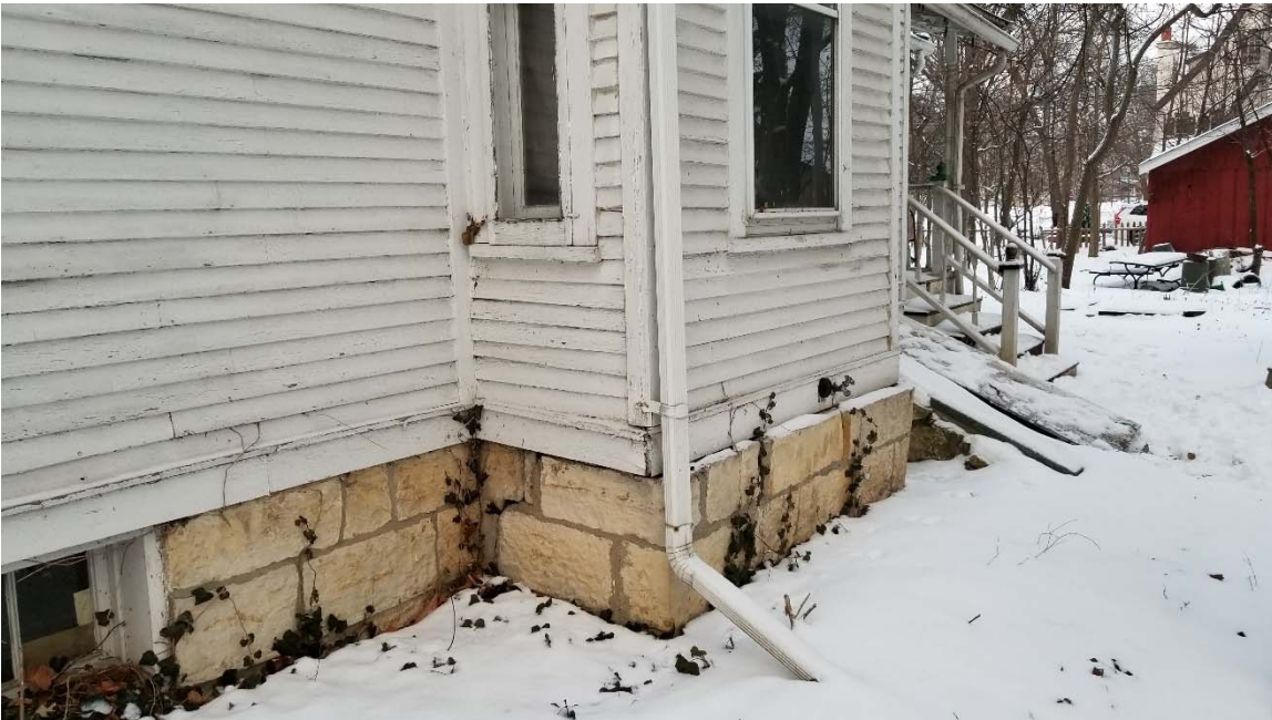
Image 12 – Bay bump out at dining room with dropped floor, walls & ceiling. Foundation cracked and pulled away from main foundation.
