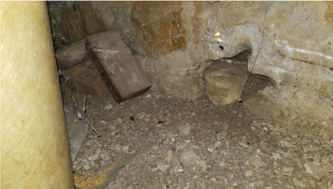
Image 17 – Stone foundation wall plugged with stone and brick with signs of water and sediment entering basement from outside.
