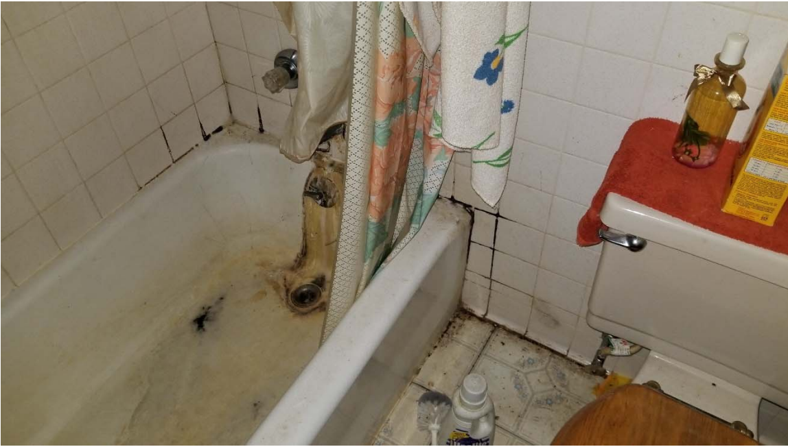
Image 5 – 2 nd floor bathroom with signs of mold
