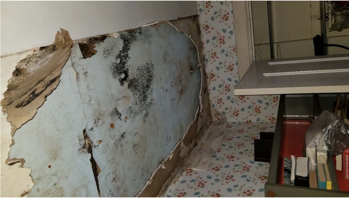
Image 7 - 2 nd floor southeast bedroom with ceiling falling in and showing signs of mold due to water damage
