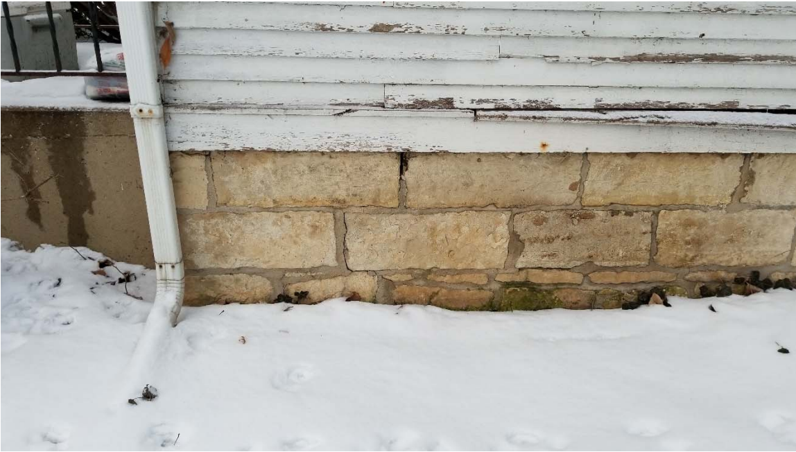
Image 21 - Stone foundation with signs of patching
