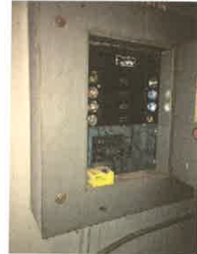
Emergency Electrical Panel Condition 1
