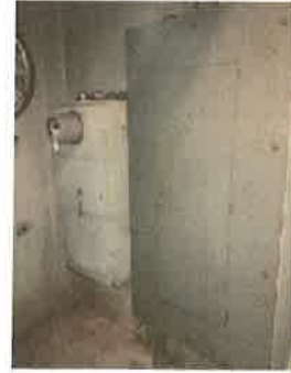
Main Electrical Service Equipment 1
