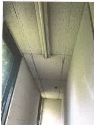
Inadequate Emergency Egress Lighting 1
