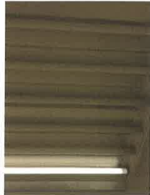
Obsolete Interior Luminaires 1
