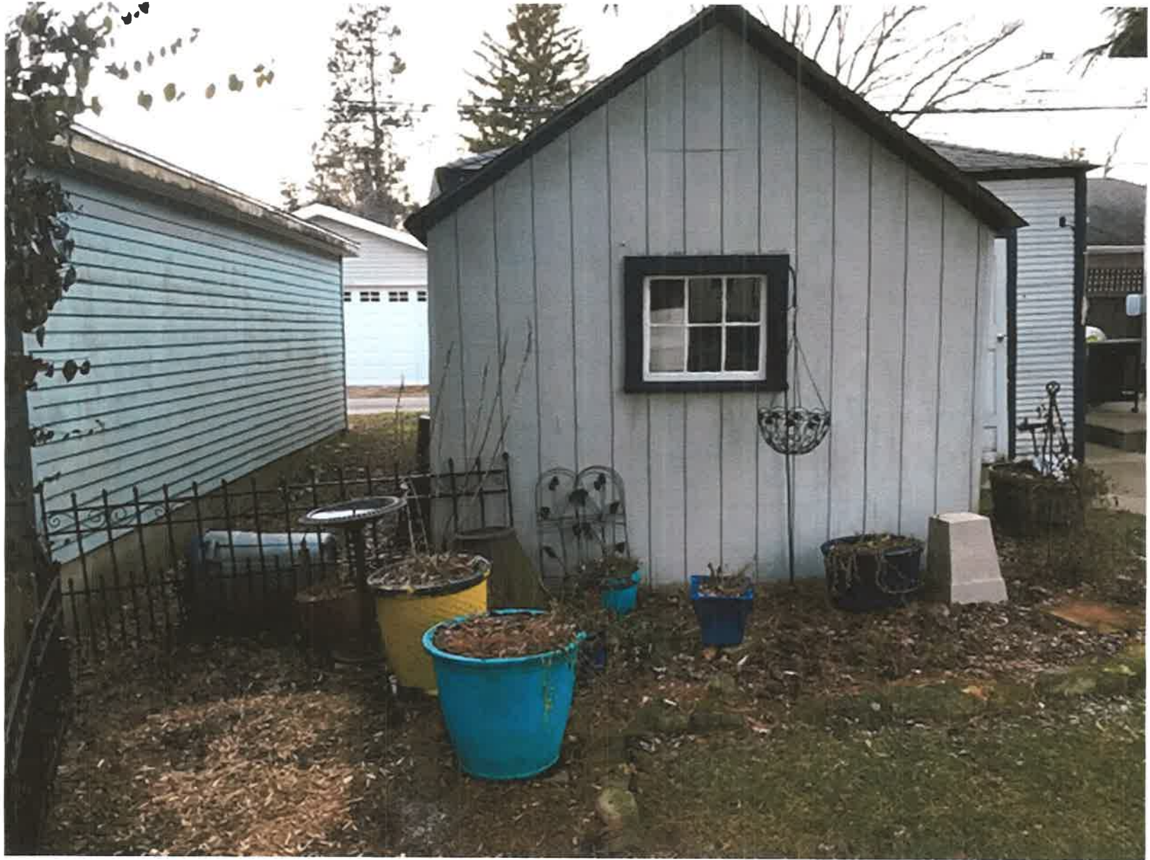
REAR OF GARAGE WITH ATTACHED SO CALLED SHED FACING EAST SHOWING SOUTH SIDE AND NORTH SIDE
