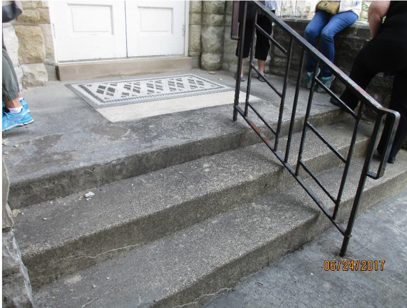
Figure 25. Isolated hairline cracks with efflorescence on stair treads and risers.
