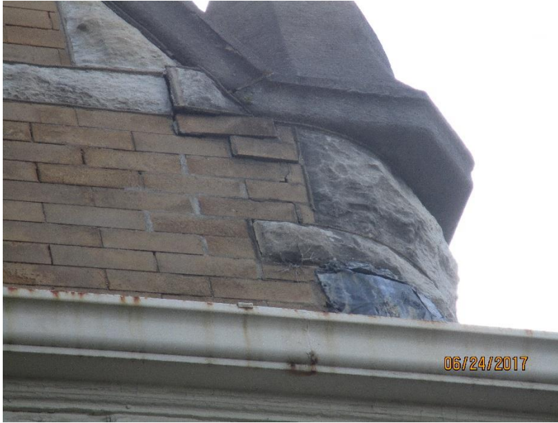
Figure 9. Detailed view of displaced brick and limestone units.
