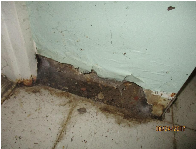
Figure 30. Moisture related distress near emergency egress door.
