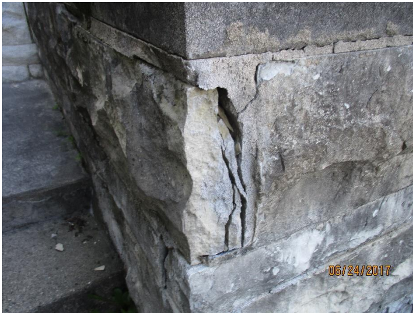
Figure 18. Detailed view of stair cheek wall cracking.
