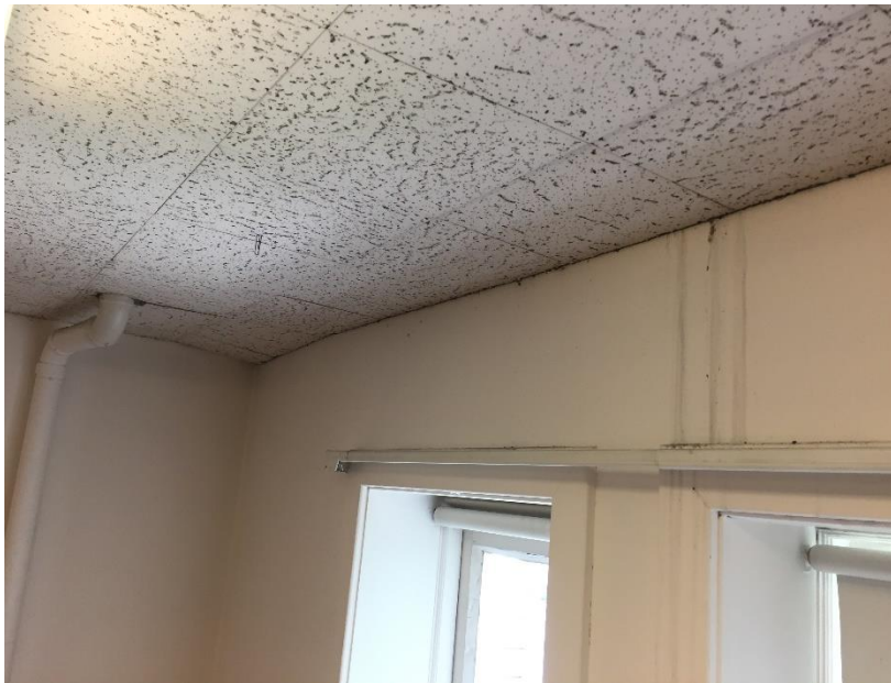
Figure 48. Interior water staining located south of the gable on the east facade.
