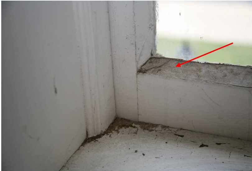
Figure 55. Second floor casement window (west facade) with putty infill replacing wood glazing stops.
