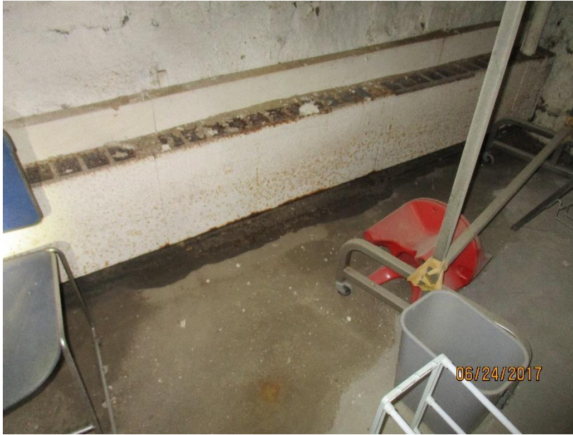
Figure 27. Evidence of isolated water infiltration at north foundation wall.
