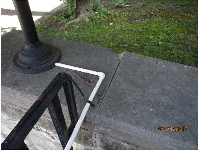
Figure 23. Open mortar joint at coping of stairway cheek wall.
