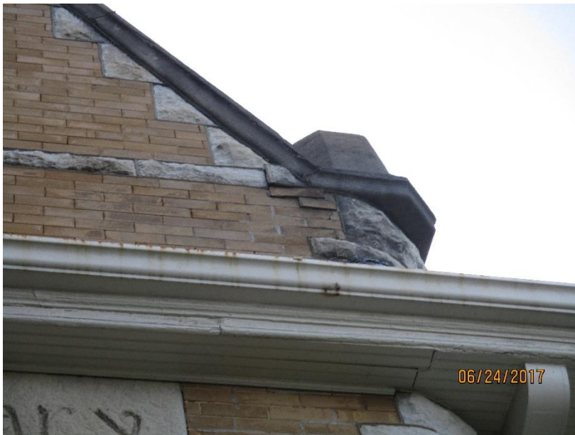
Figure 8. General view of isolated displaced brick and limestone.
