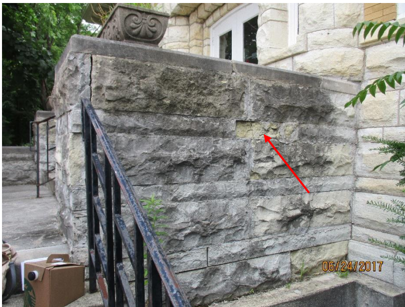
Figure 22. Additional view of scaling/spalling of face-bedded stone.
