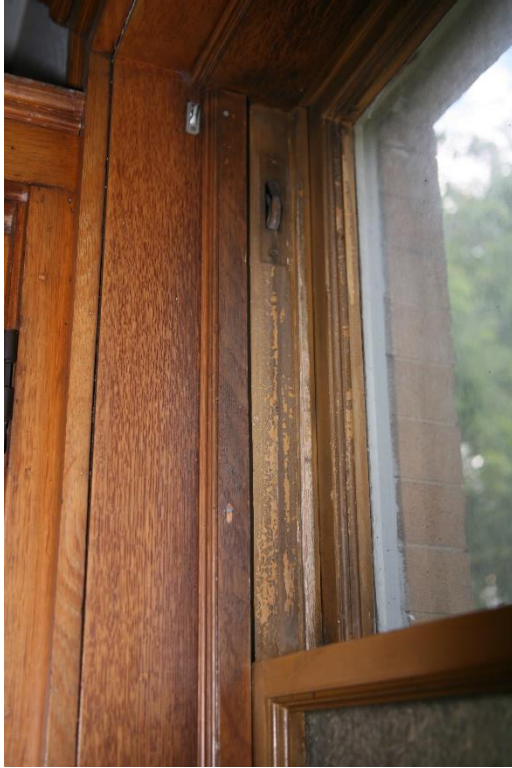
Figure 59. View of window with missing sash cord.
