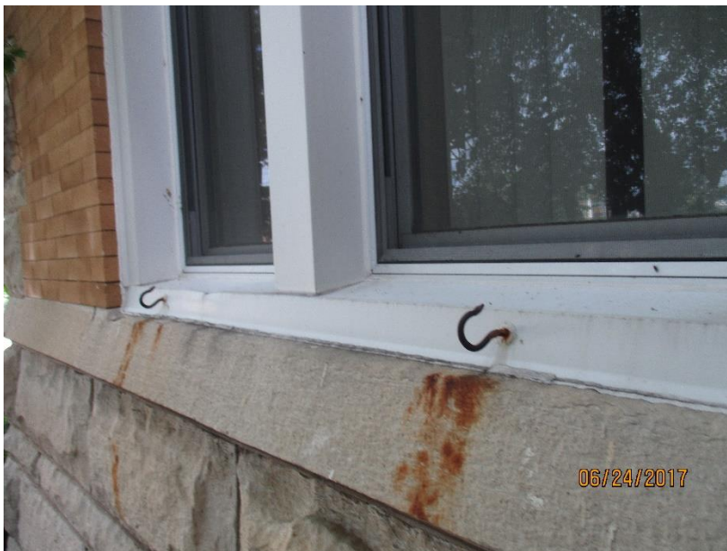
Figure 14. Note corrosion staining.
