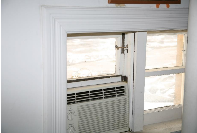
Figure 57. Window sash modified to accommodate A/C unit.
