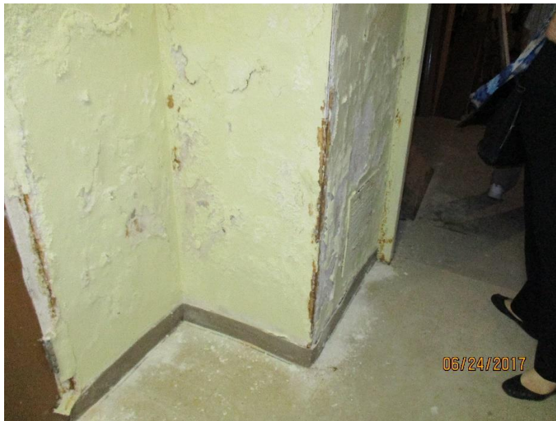
Figure 32. Moisture related distress evident on plaster wall.
