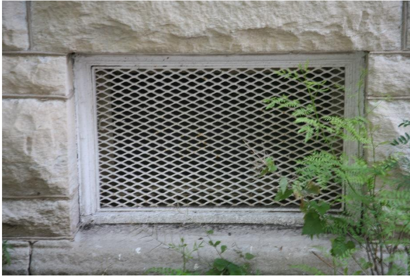
Figure 62. Typical basement window covered with metal screening.
