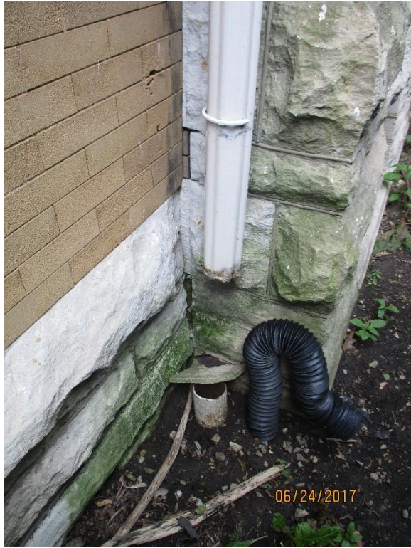
Figure 15. Minor biological growth present on rusticated stone and improperly detailed downspout at northwest corner of the building.
