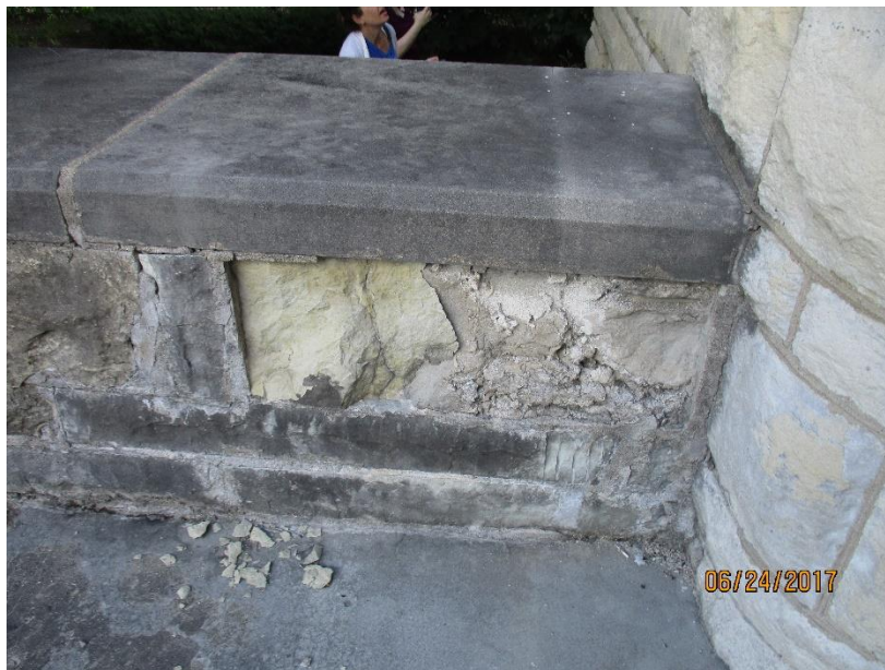
Figure 20. Scaling and spalling of face bedded stone at stairway cheek wall.
