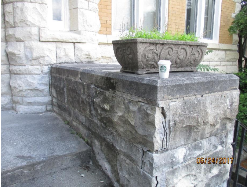
Figure 17. Isolate mortar cracks in stairway cheek walls.
