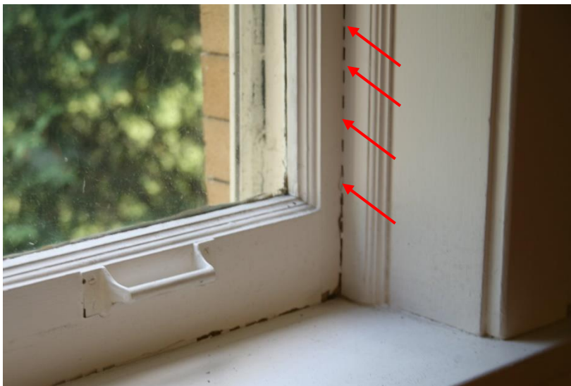
Figure 58. Arrow indicates bridges of paint fixing the lower sash in closed position.
