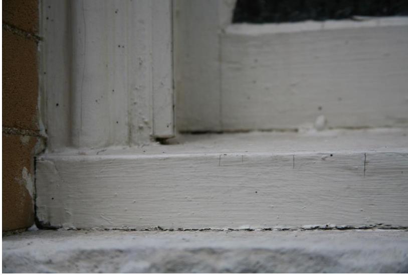
Figure 53. No observed perimeter sealant at connection of wood and stone sill.
