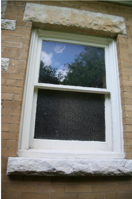
Figure 49. View of typical wood double-hung window. This window includes privacy glass in the lower sash.
