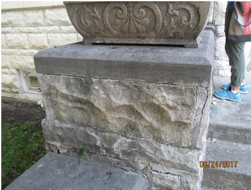
Figure 24. Cracked and debonded mortar between stone units.
