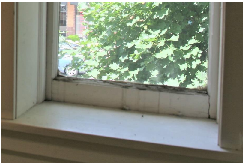
Figure 50. View of most distressed interior paint observed.
