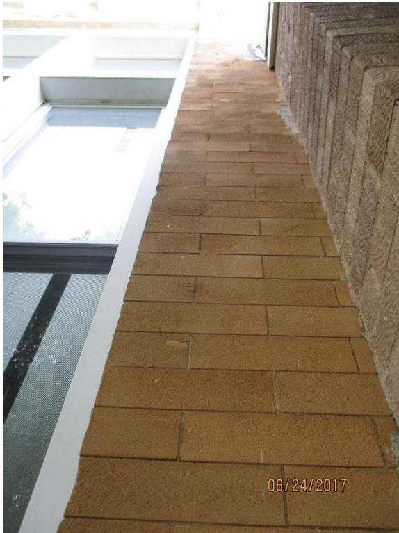
Figure 10. Locations of minor mortar erosion.
