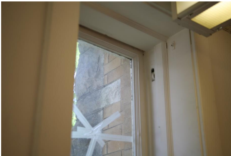
Figure 56. View of cracked glass.
