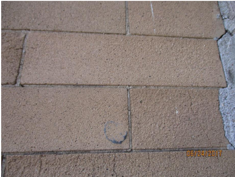
Figure 12. Note brick texture roughened due to sandblasting.
