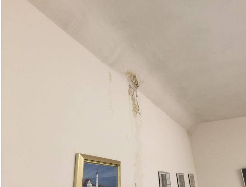
Figure 47. Interior water staining corresponding to vent stacks on east roofing area, north of the dormer.
