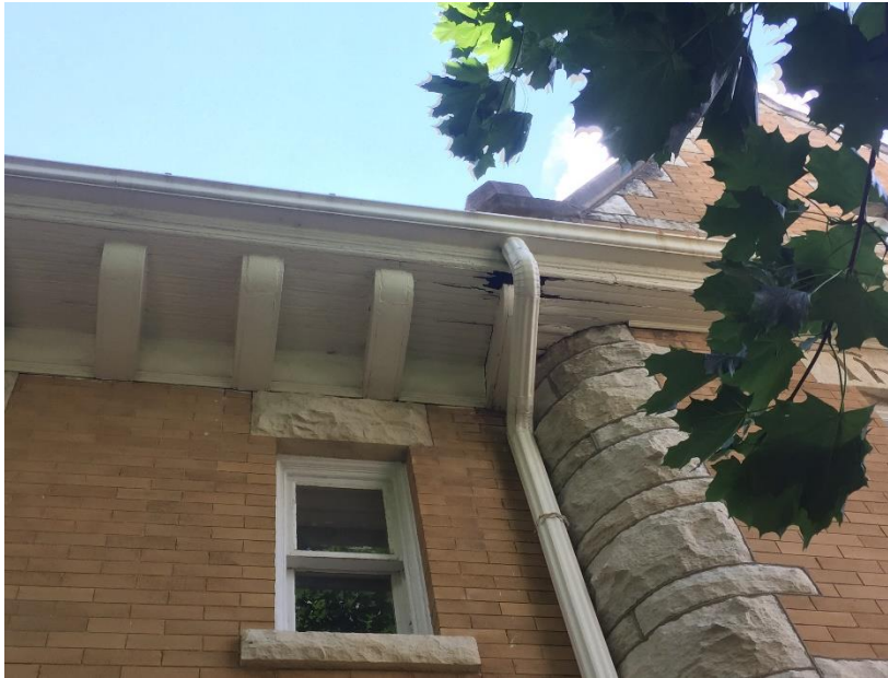
Figure 43. Isolated wood deterioration and peeling paint at soffit and fascia.
