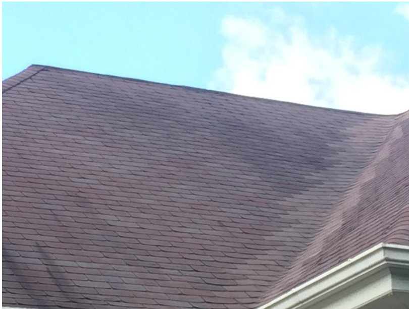
Figure 40. Location of previous ridge repair.
