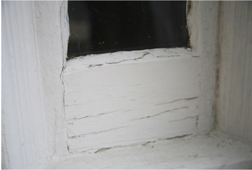
Figure 51. View of exterior of wood window with paint distress (more significant than most) and cracked glazing putty.
