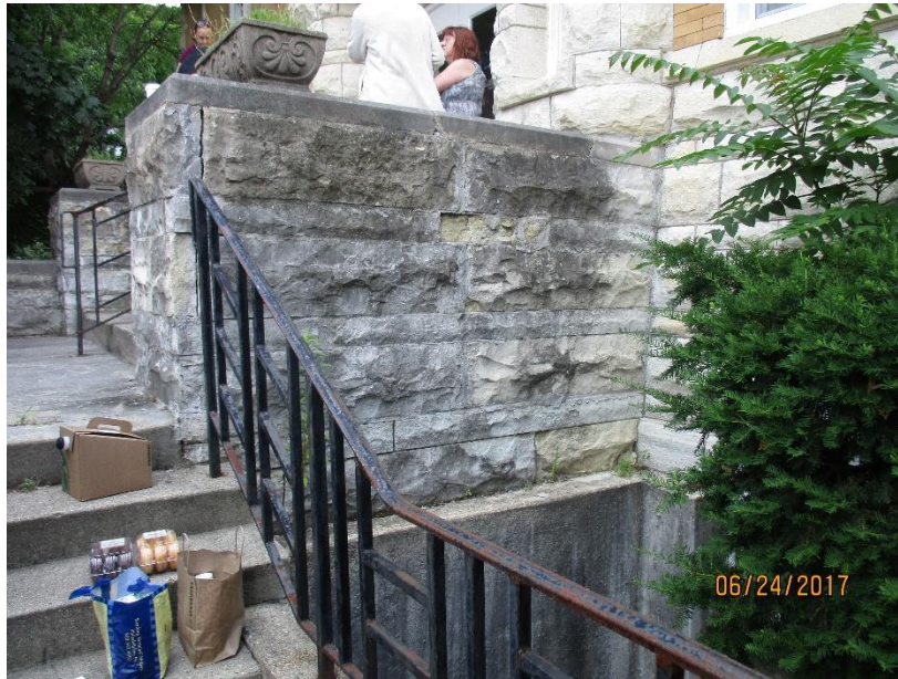
Figure 19. Alternate view of isolated stair cheek wall cracking.
