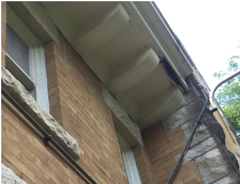
Figure 44. Opening in soffit at the east side of the gable on the north facade.
