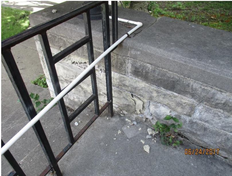
Figure 21. Additional view of scaling/spalling face-bedded stone.
