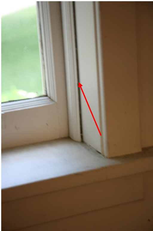
Figure 54. Gap between interior wood stop and window frame.
