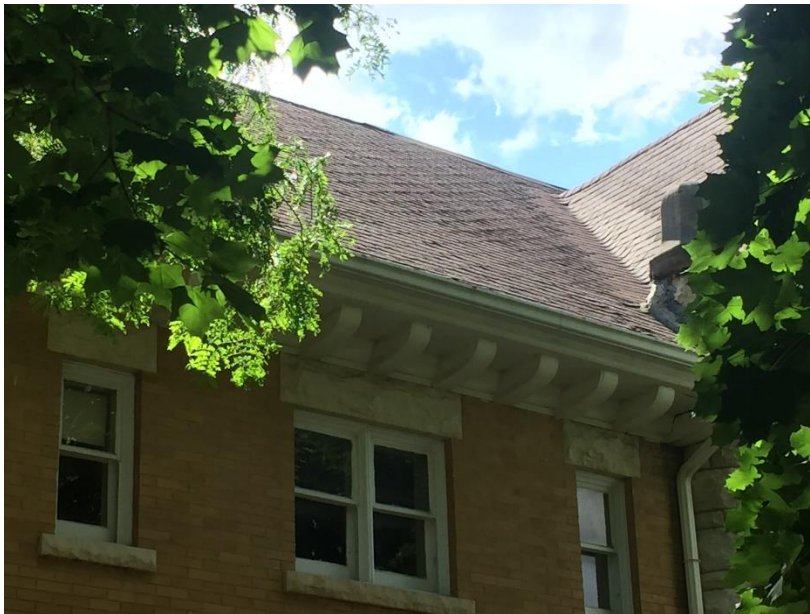
Figure 38. General view of curling/cupping of shingles.
