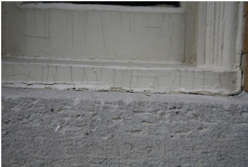
Figure 52. Cracked/debonded perimeter sealant at connection of wood and stone sill.
