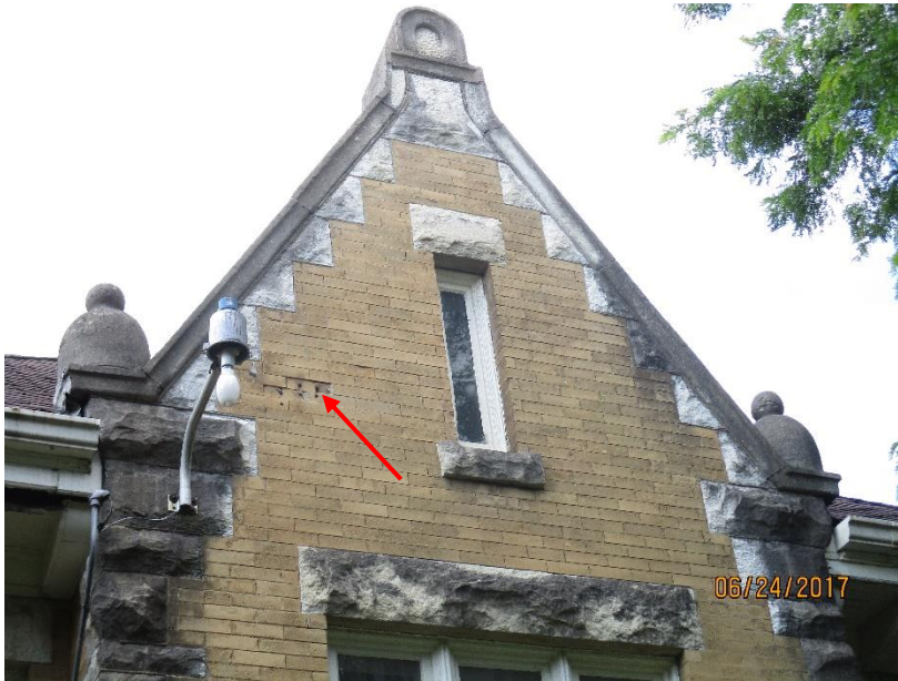
Figure 13. Note spalls at locations previously used for anchorage.
