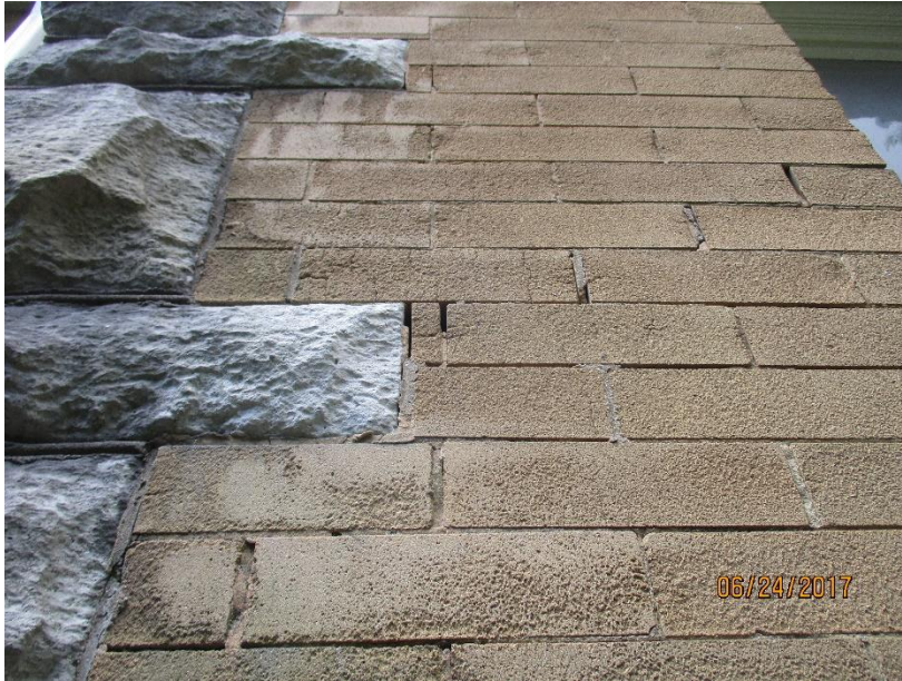
Figure 11. Locations of minor mortar erosion.
