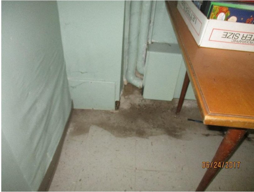
Figure 29. Evidence of moisture, potentially from nearby radiator.
