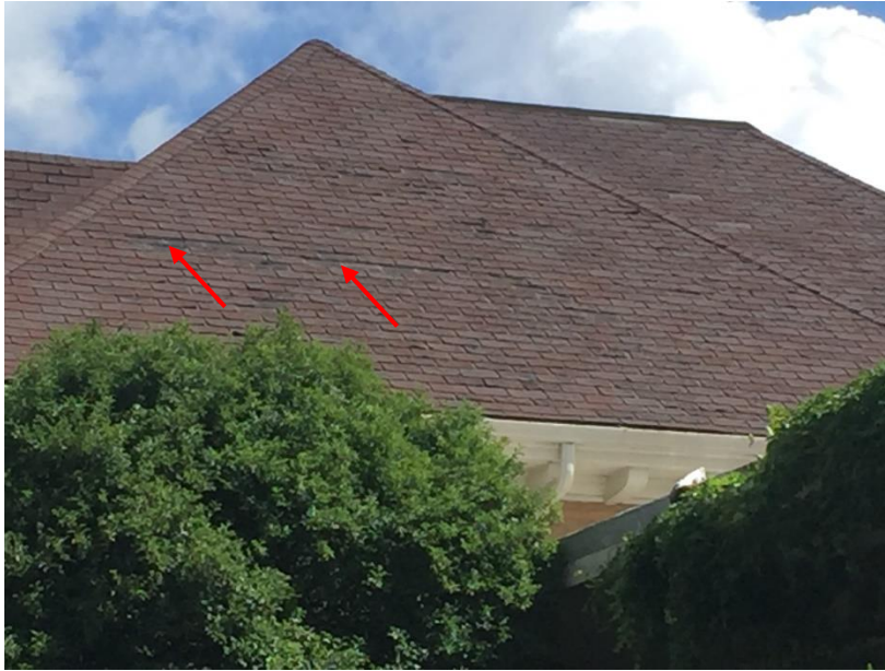
Figure 39. General view of south roofing area with areas of missing shingle tabs.
