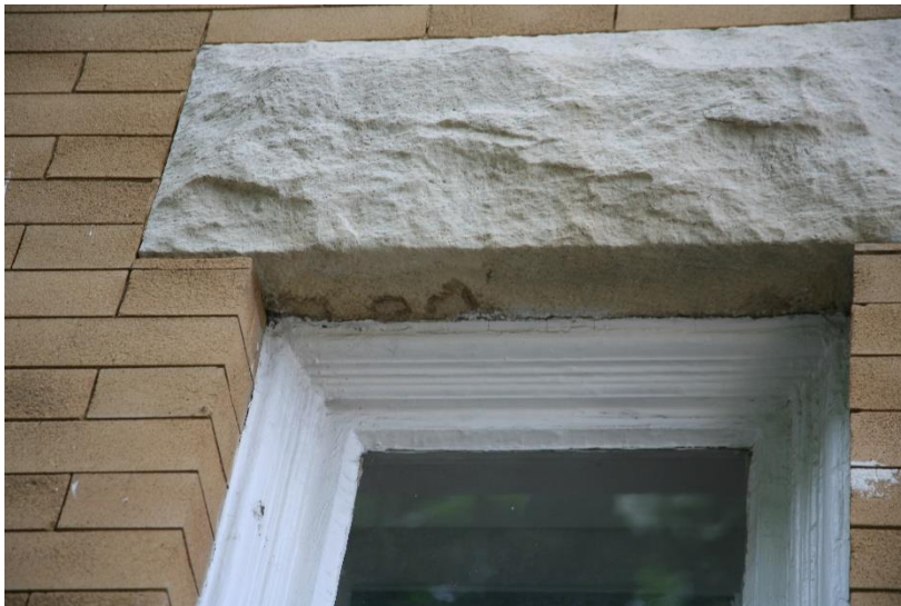
Figure 61. View of staining due to watershed patterns on the window lintel.
