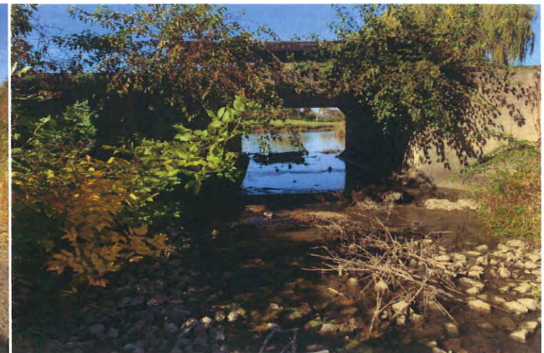
A concrete weir and box culvert was observed within Clow Creek on the West property line.
