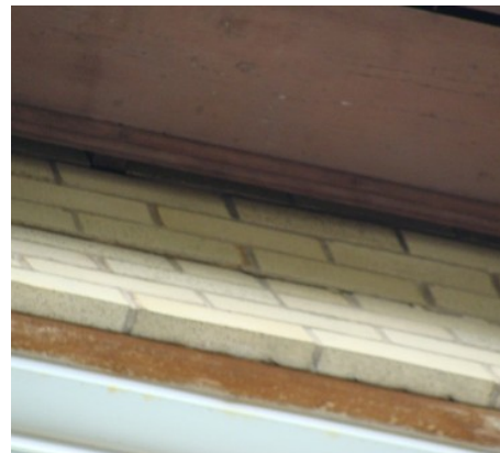
Photo #2 – Displaced brick at eave on west face of 619
