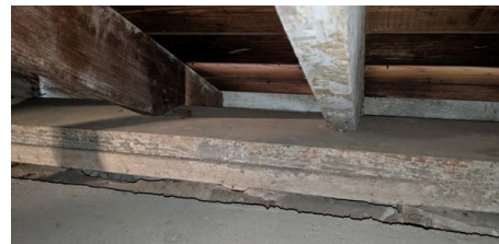
Photo #4 – Displaced Rafter Plate at top of west wall of 619
