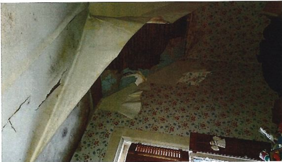
Image 6 – 2 nd floor southeast bedroom with ceiling falling in and showing signs of mold due to water damage
