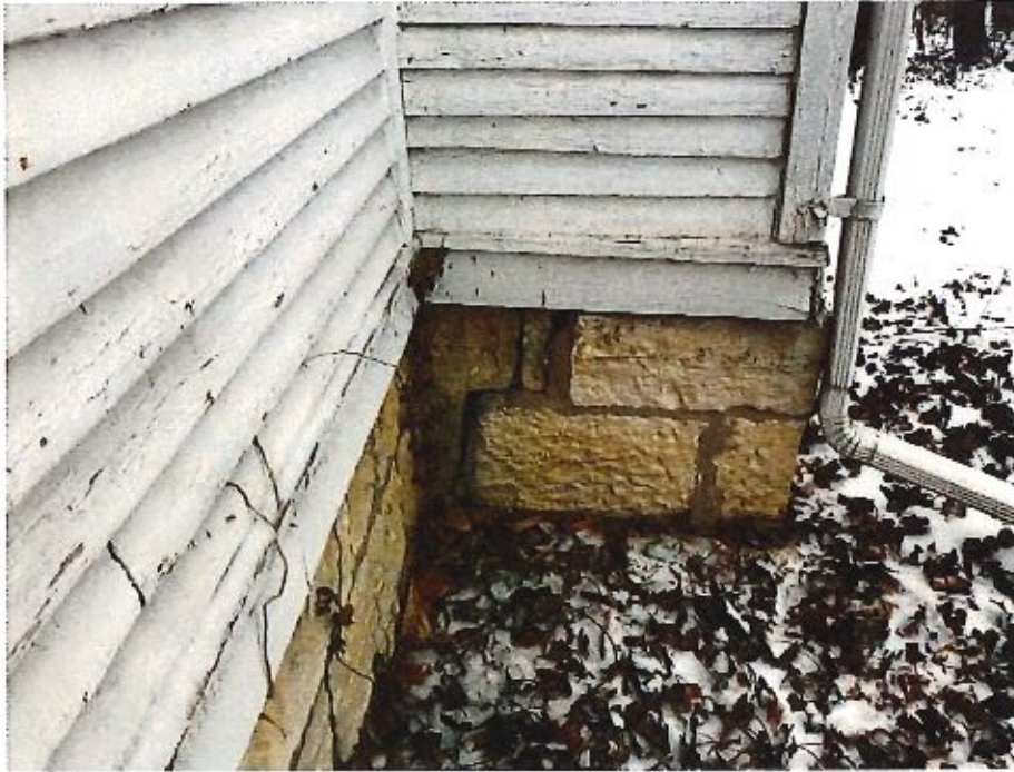
Image 10 – Leaning wall at stair
