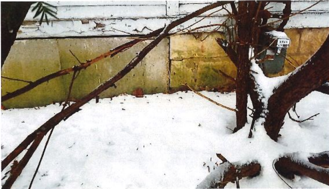
Image 9 – Concrete foundation dropped or settling at stone foundation. Stone foundation has signs of cracking also.
