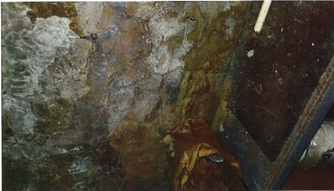
Image 16 – Stone foundation joints patched and if rubbed with finger, is rubs off as can be seen with sand sitting on wood ledge.
