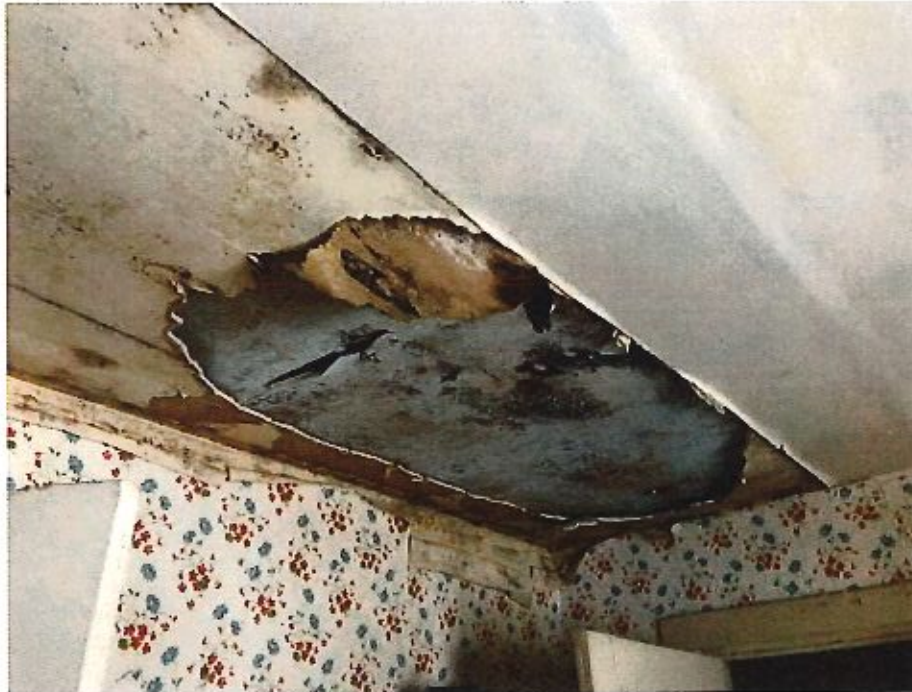
Image 11 – Water damage on second floor ceiling
