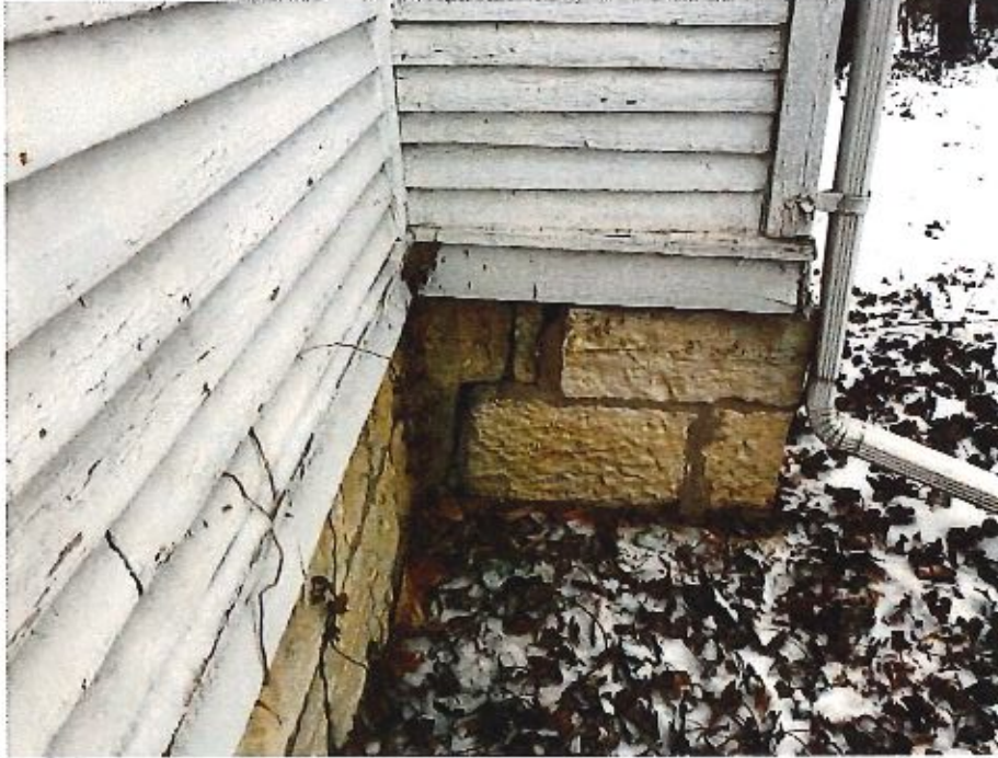
Image 10 – Leaning wall at stair
