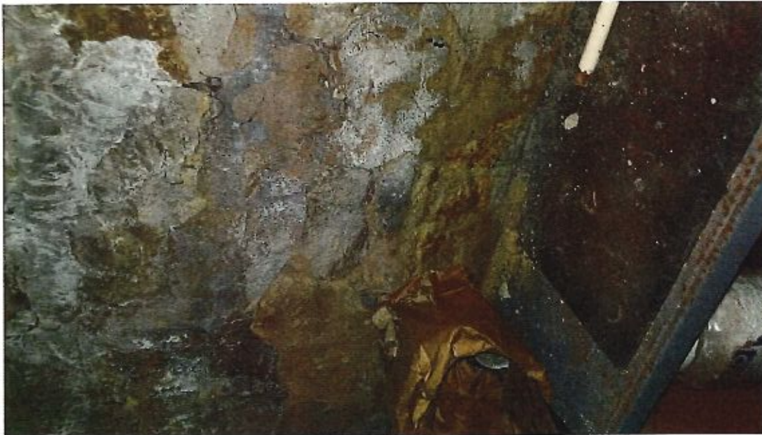
Image 16 – Stone foundation joints patched and if rubbed with finger, is rubs off as can be seen with sand sitting on wood ledge.
