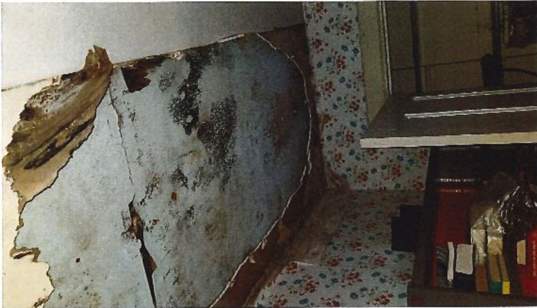
Image 7 - 2 nd floor southeast bedroom with ceiling falling in and showing signs of mold due to water damage
