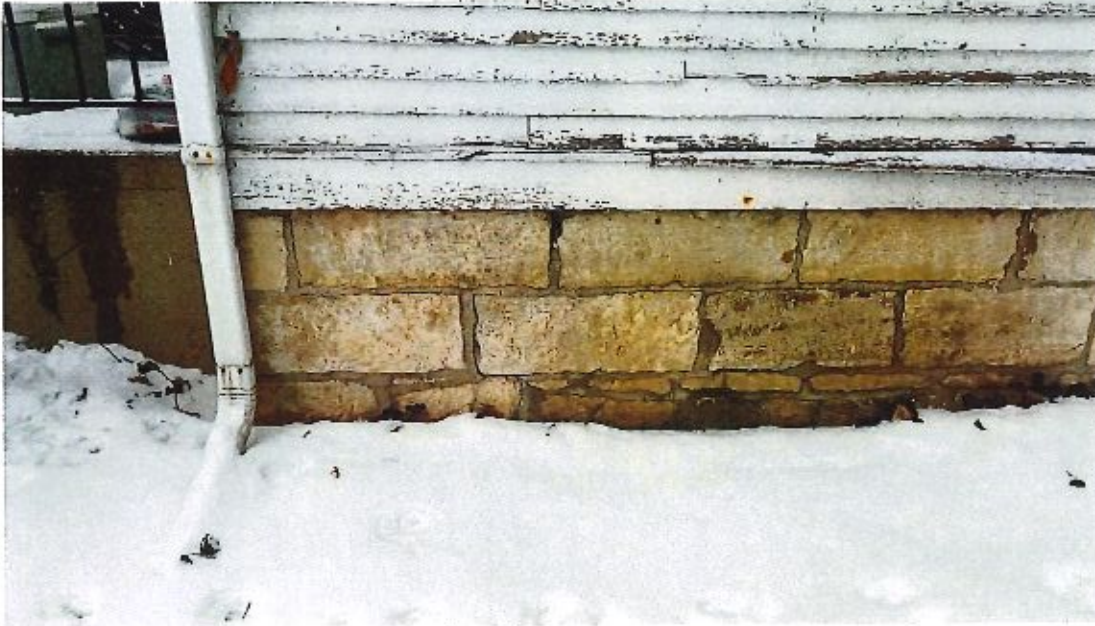
Image 21 - Stone foundation with signs of patching
