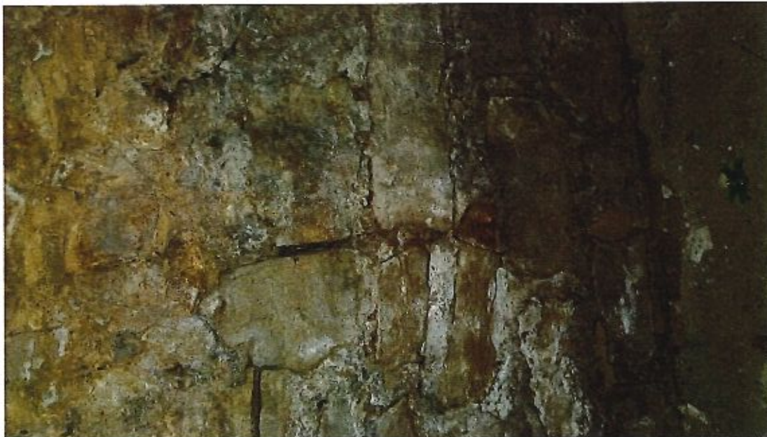
Image 18 – Stone foundation cracks with signs of seepage.
