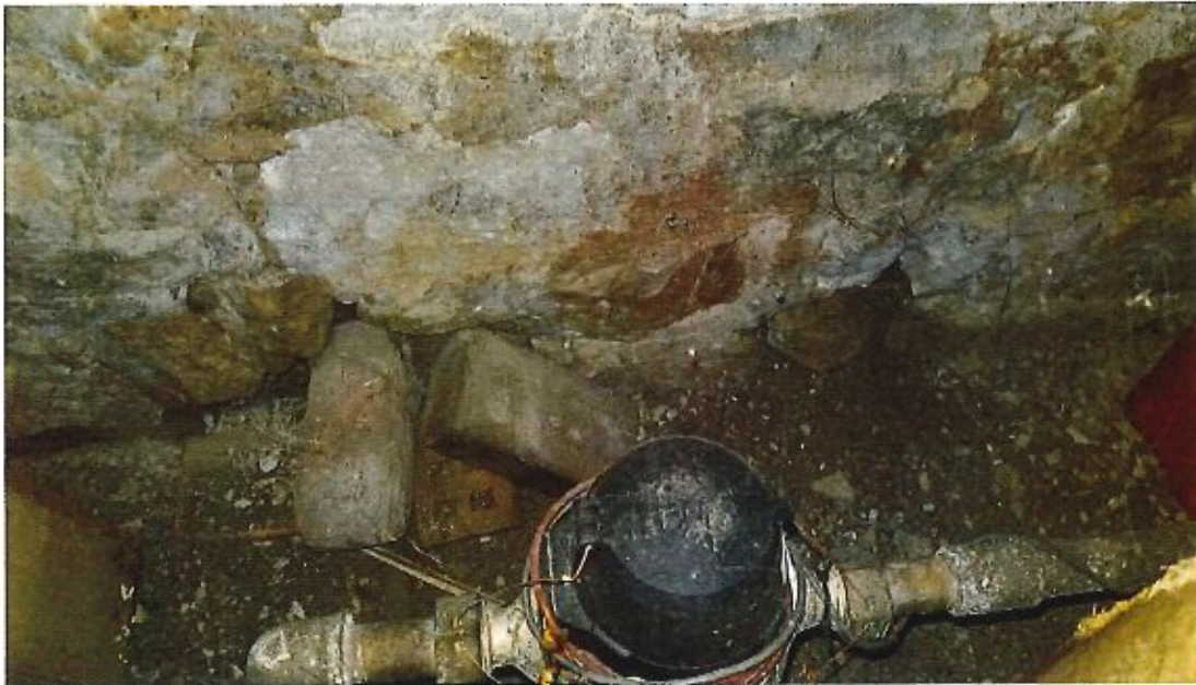
Image 13 – water meeting with copper connections to lead water piping. Also, bottom of wall where bricks and stones located have holes where water and debris is filtering into basement.
