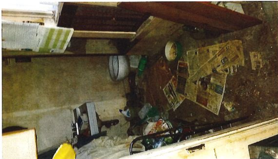
Image 4 – First floor bathroom with filth and signs of mold around toilet.
