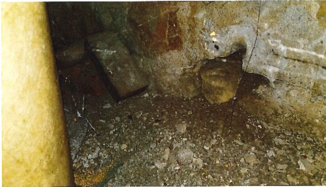
Image 17 – Stone foundation wall plugged with stone and brick with signs of water and sediment entering basement from outside.
