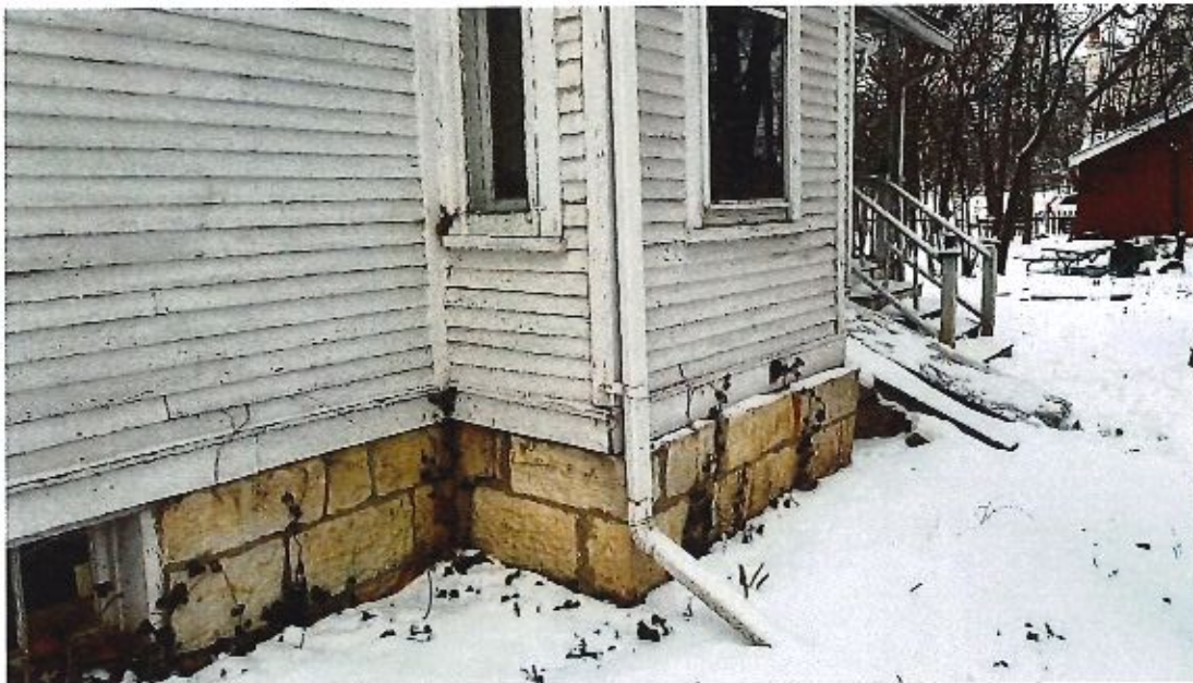
Image 12 – Bay bump out at dining room with dropped floor, walls & ceiling. Foundation cracked and pulled away from main foundation.
