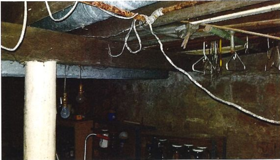
Image 15 – Undersized basement wood beam with lights hanging from ceiling with rope cord
