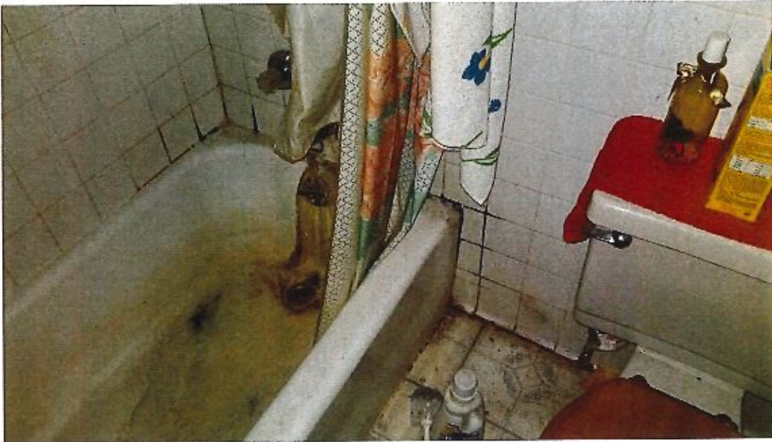
Image 5 – 2 nd floor bathroom with signs of mold
