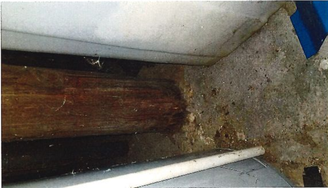
Image 23 – Rotting wood post in basement supporting middle beam
