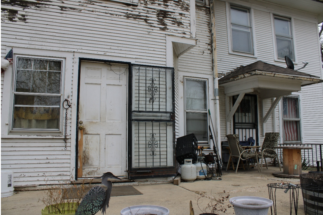
Detail of rear façade showing doors to kitchen (left) and to southwest room (right).
