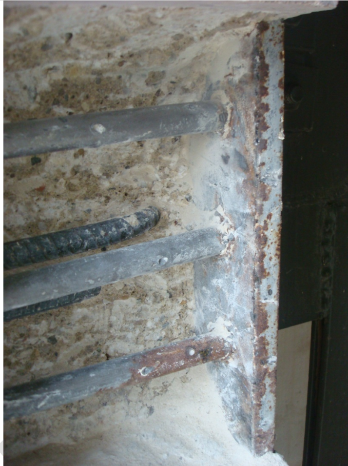
Photograph #6: Backside of connection plate and embedded studs at northeast side of Elev. 52.5.
