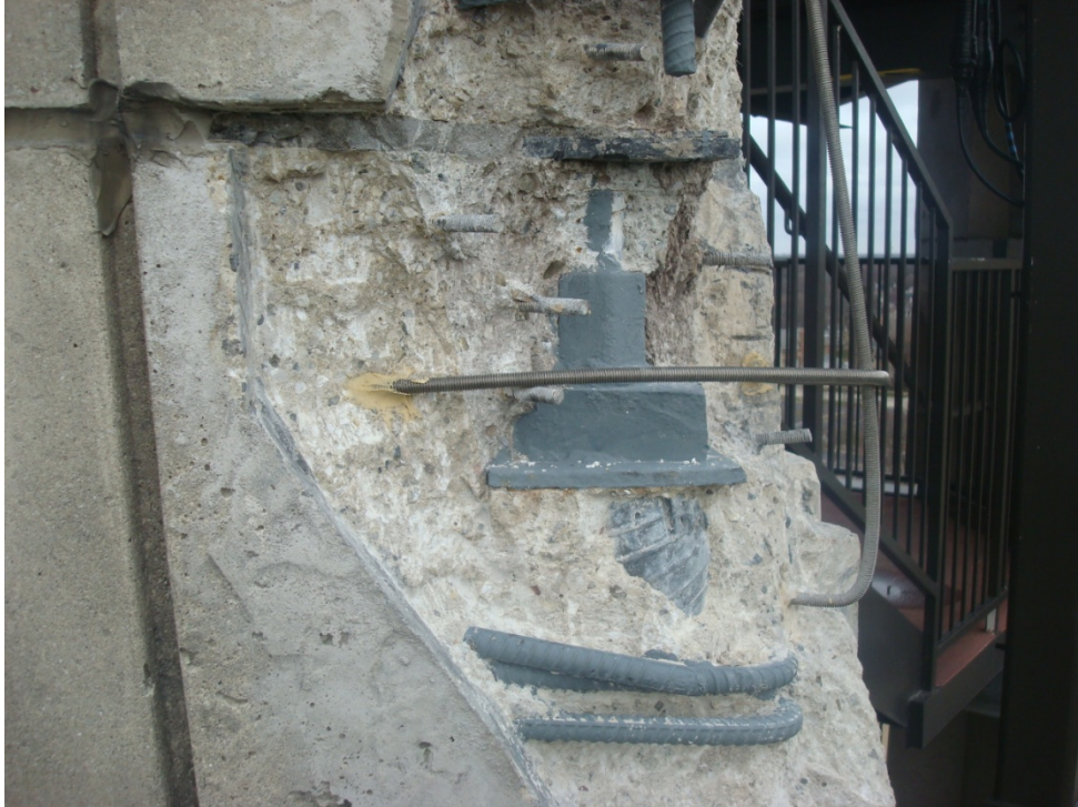
Photograph #4: Exposed end of PT rod and reinforcement bars at right opening
