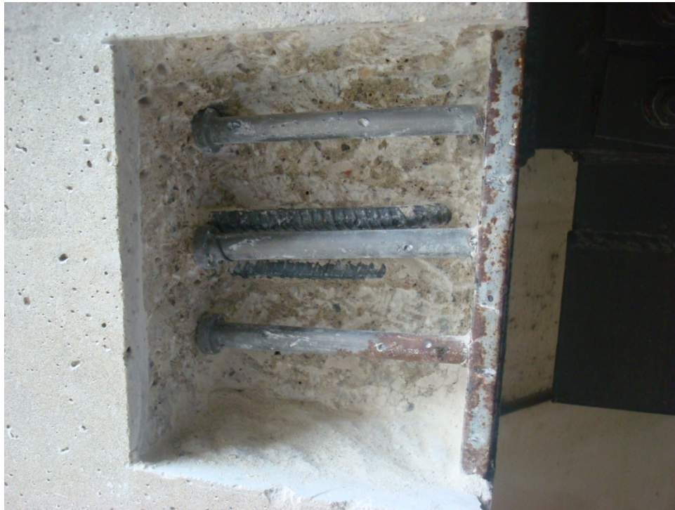
Photograph #5: Exposed connection plate and embedded studs at northeast side of Elev. 52.5.
