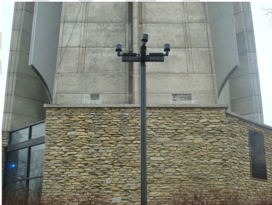
Photograph #1: Areas of exposed post-tensioned rods at NW corner.
