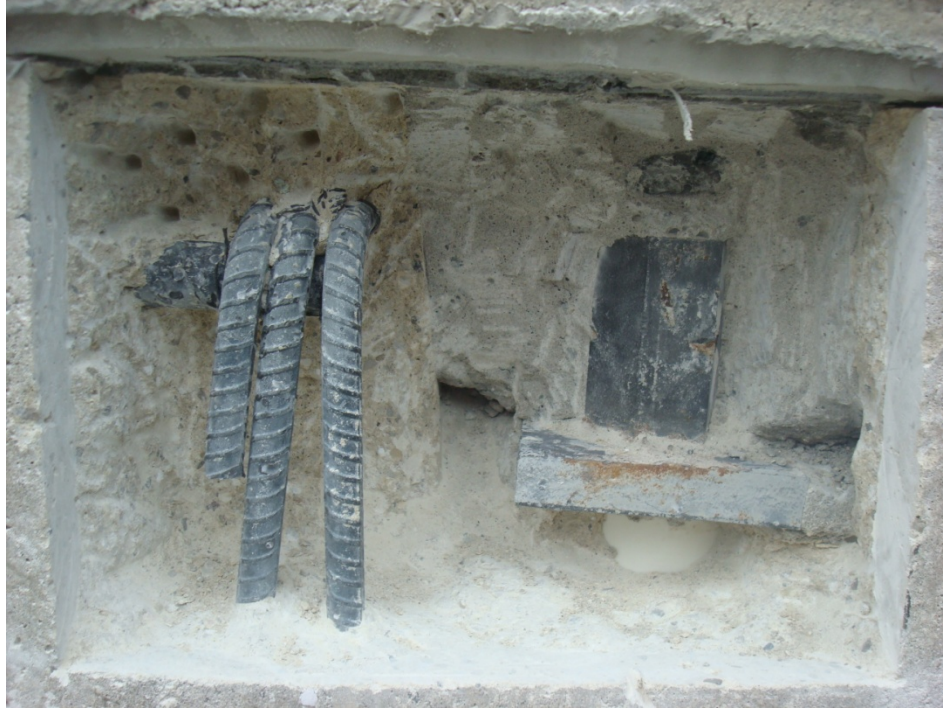
Photograph #2: Exposed end of PT rod and reinforcement bars at left opening
