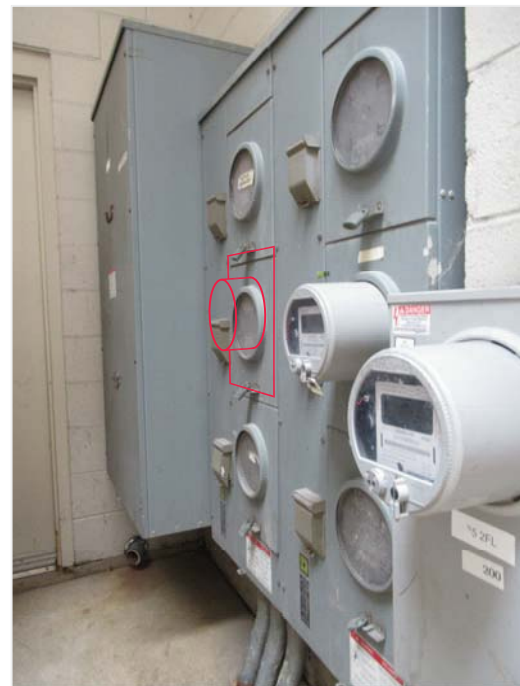
PROPOSED ELECTRICAL SERVICE METER TO BE INSTALLED AT EXISTING MULTI-GANG METER BANK NEAR EXISTING TRANSFORMER
