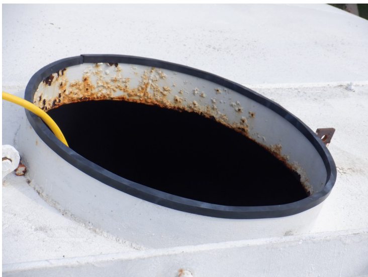
51) A gasket was installed on the wet interior hatch by Dixon during the inspection.
