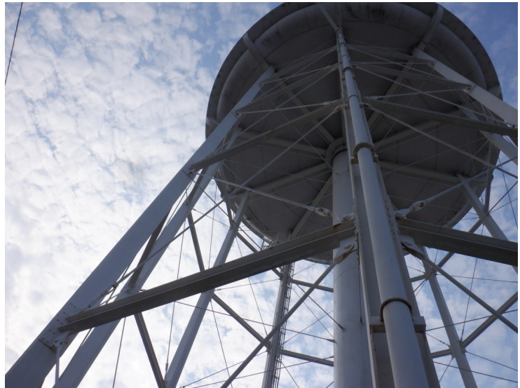
17) The leg coating is in fair condition overall.
