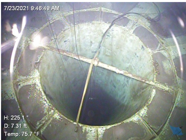
66) There is no safety grate over or around handrail the riser.
