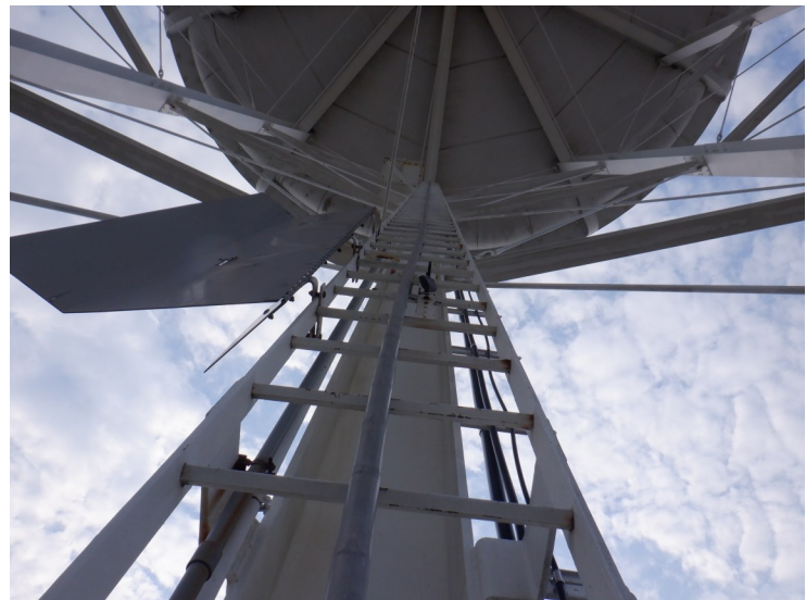
20) The ladder is in good condition. The ladder is equipped with a fall prevention device.
