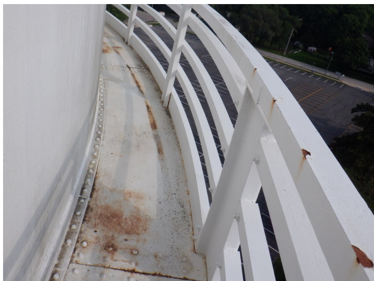
33) Spot coating failures on the handrail.
