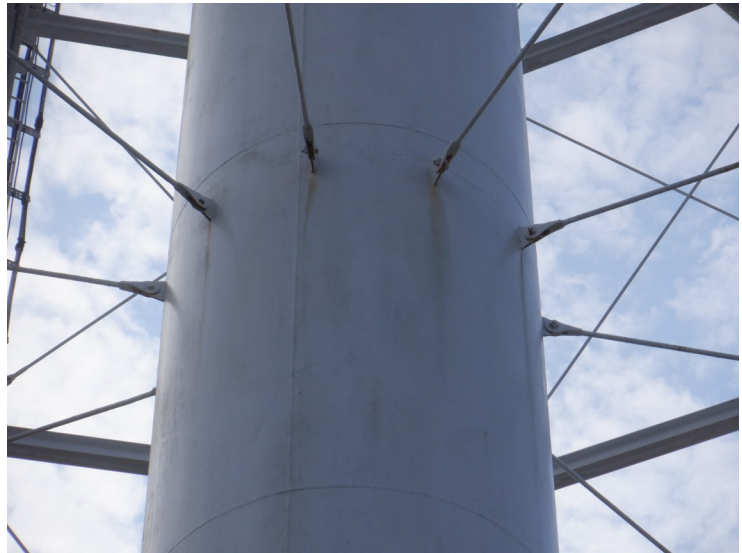
8) The riser tie rods are attached to welded lugs that are in good condition.
