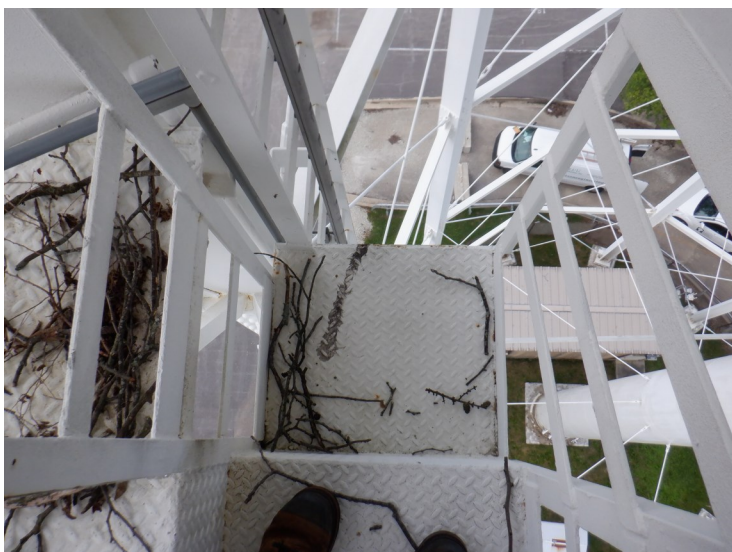
24) The step-off platform under the bowl is in good condition. There are remains of a hawk nest on the platform.
