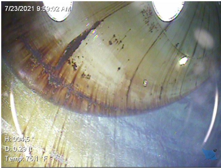
55) Spot coating failures on the wet interior sidewall.
