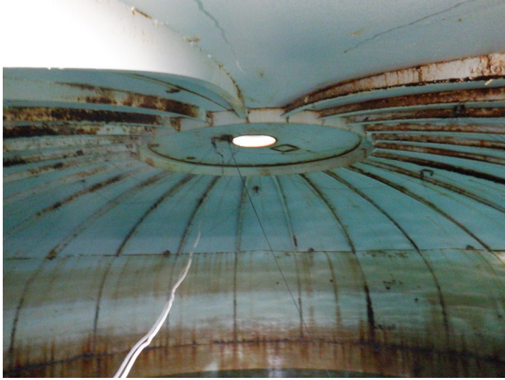
52) The wet interior roof coating is in poor condition overall.
