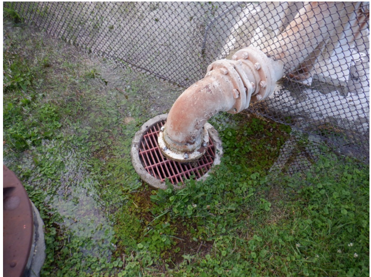
14) The overflow pipe discharges to a catch basin.
