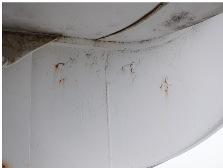
27) Spot coating failures on the radial arm bowl stiffeners.
