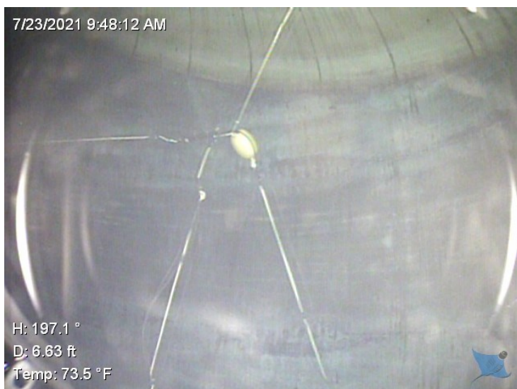
60) The floating ring cathodic protection system appears to be in good condition.
