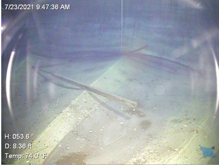
64) The painter's railing has broken from the sidewall and is lying on the bowl.
