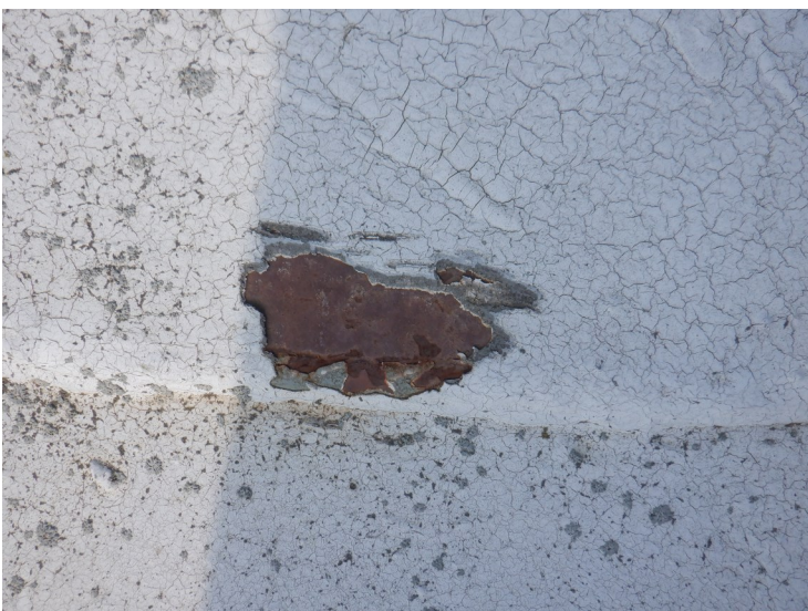
48) Spot coating failure on the roof.
