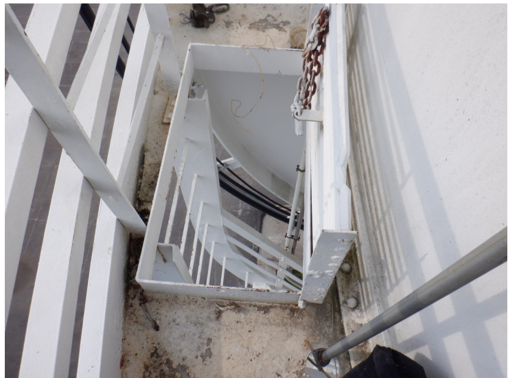
29) The balcony ladder opening is in good condition. The opening cover is in good condition.
