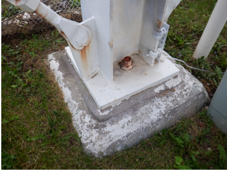
10) Typical leg foundation that is in good condition. The coating is in poor condition overall.
