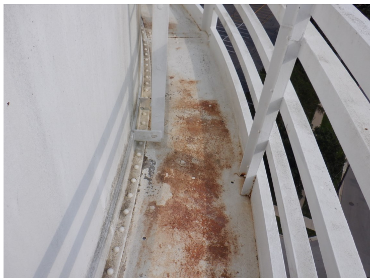
30) The balcony is in good condition. The coating is in poor condition.
