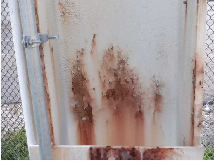
16) Coating failures with rust undercutting on a leg.
