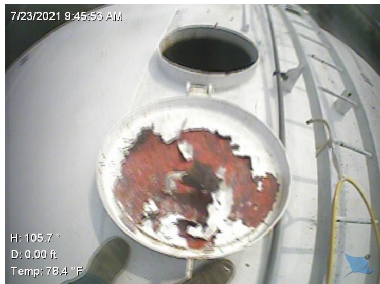
50) The wet interior roof hatch is in good condition. There are spot coating failures on the cover.
