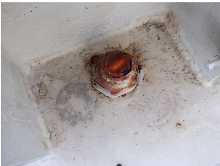
12) Anchor bolt with minor steel loss from corrosion.
