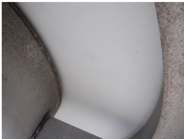
42) The vent pressure plate is in good condition and was found to be properly aligned during the inspection.
