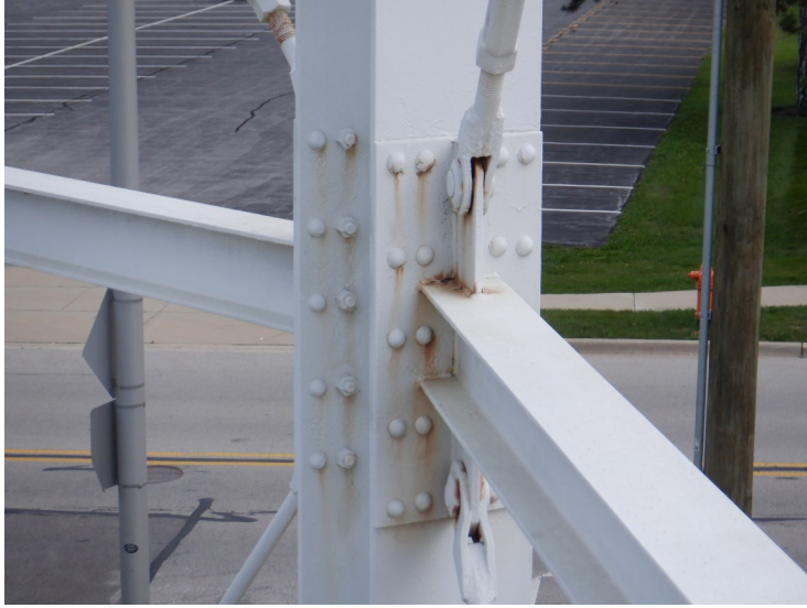
22) Spot coating failures and rust bleedthrough at a strut and leg connection.
