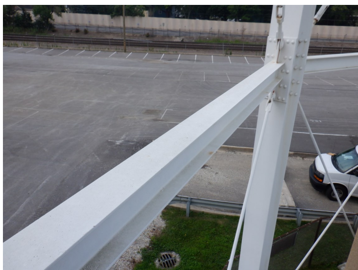
21) Typical strut section that is in good condition. The coating is in fair condition overall.
