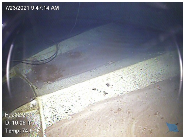
62) The bowl coating is in fair condition overall.
