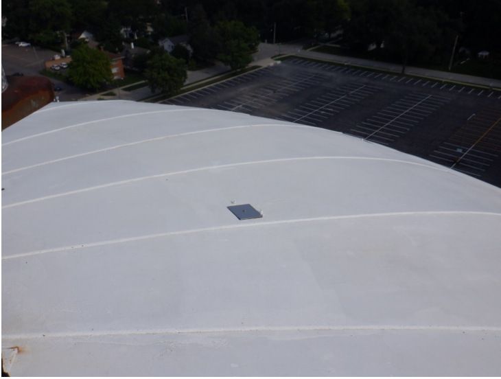
46) The roof coating is in poor condition overall.
